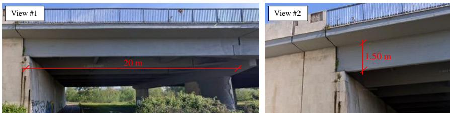
Fig. 4 Details of investigated span (adapted from https://maps.app.goo.gl/BYHCM9kHMvgMR-BiU8 ); span length on the left (View #1), cross-section height of the beam on the right (View #2).
