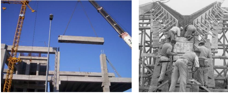
Fig. 1 e 2 Construction site machinery in the assembly of a building using simple schemes of precast reinforced concrete elements, 2012; Labor force in the construction of the Palazzetto dello Sport in Rome designed by P.L. Nervi, 1956.
