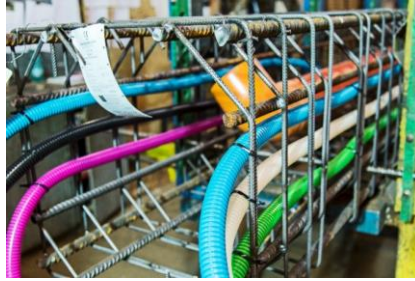
Fig. 1 Sensors and pipes installed over the reinforcement cage of a smart column at one of the Manini production plants
